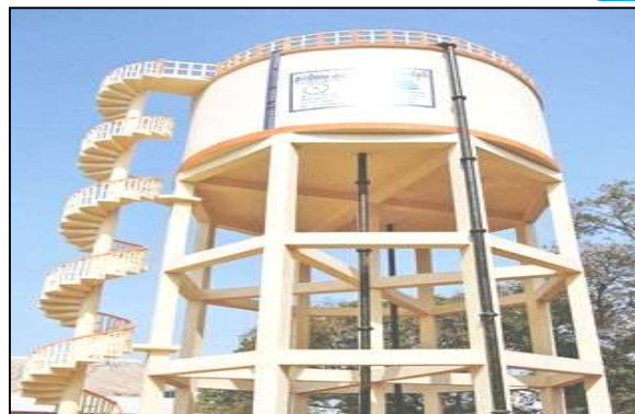
Water distribution tank
