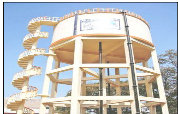
Water distribution tank
